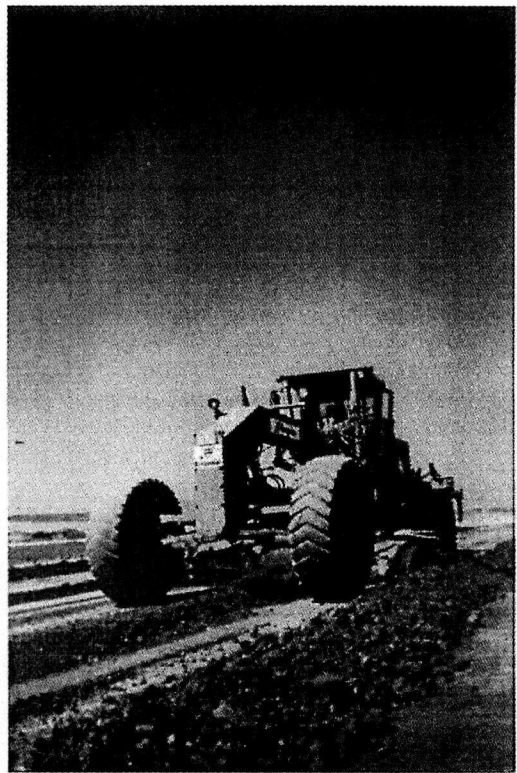
Fig. 2: Panoramic view earthworks using the laser system with motor grader, emitter and target levelling-rod.
