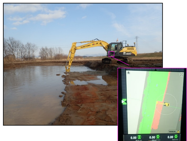
Figure 5. ICT construction (3D-machine control) (Appearance Guidance and the monitor which shows the excavation status in operation room)
