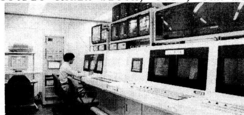
Photo 20. Internal appearance of the control room
