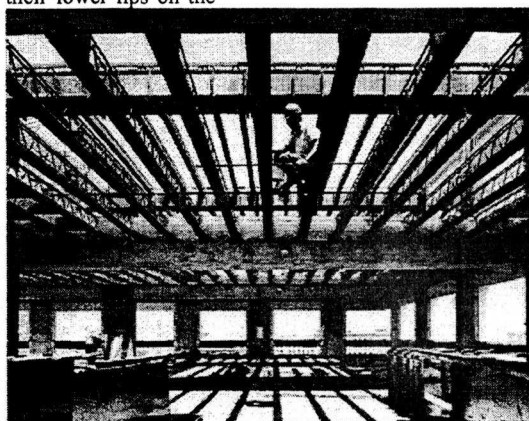
Fig 2 - A general view of a high rise office structure being constructed by the PS method
