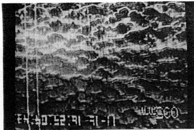
FIG. 9 IN-PIPE LINING CONDITIONS
