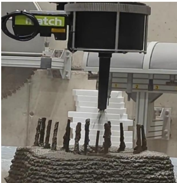
Figure 1. Shotcrete 3D Printing (SC3DP) at the DBFL of the ITE TU Braunschweig including short reinforcement bar insertion, as proposed by Dörrie et al. [7], and a 2D laser profiler running ahead of the printing nozzle. The goal of our paper is the detection of the depicted type of reinforcement elements.
