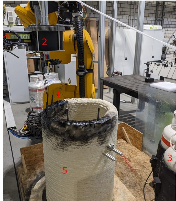
Figure 5. Foam printing test bench at Institute of Assembly Technology and Robotics. 1) printing robot 2) printing head including nozzle and slip ring 3) material supply 4) sensor-module 5) printed column with colouring and rebar integration
